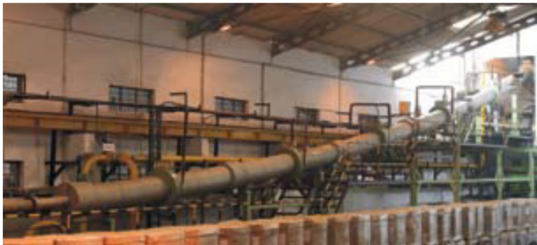
Two C. C. V. Line for XLPE Cables upto 132 kv
